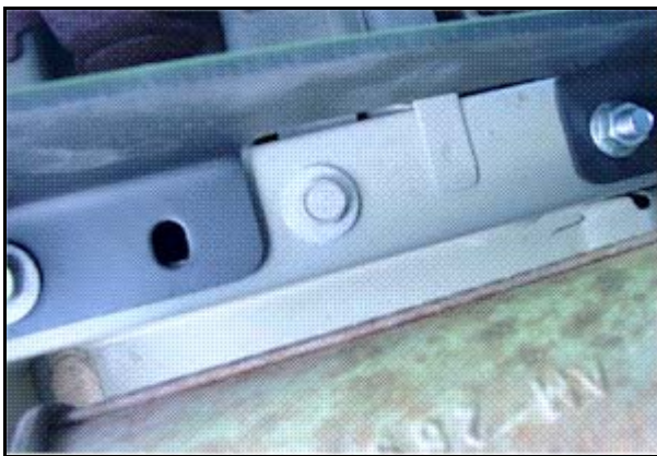
We bolted up the hitch to the frame and the new bolts.
